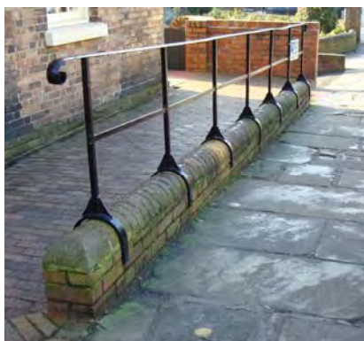
7a. Alternative wrought iron rail, as part of railing, fixed to low wall
