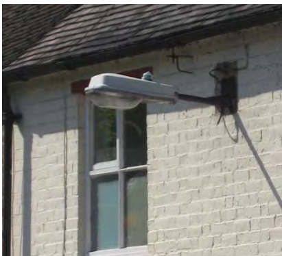
9a. Wall mounted street lighting
